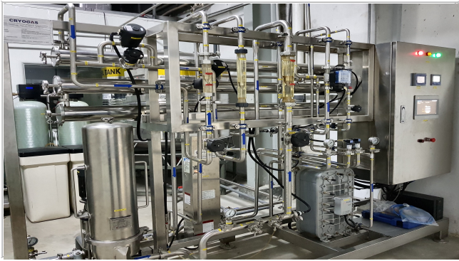
Figure 1. Purified Water Generator skid
